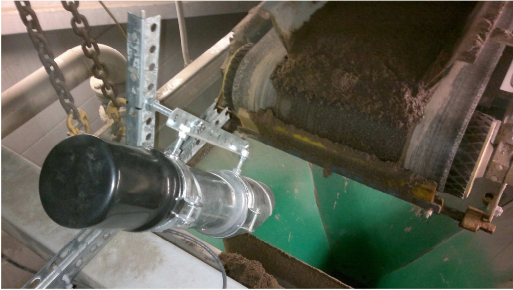
Fig. 1. WCM411 moisture sensor installed over a silo belt feeder to measure dropping aggregate. The sensor is located in the black plastic hat at the upper end of the protection tube.
