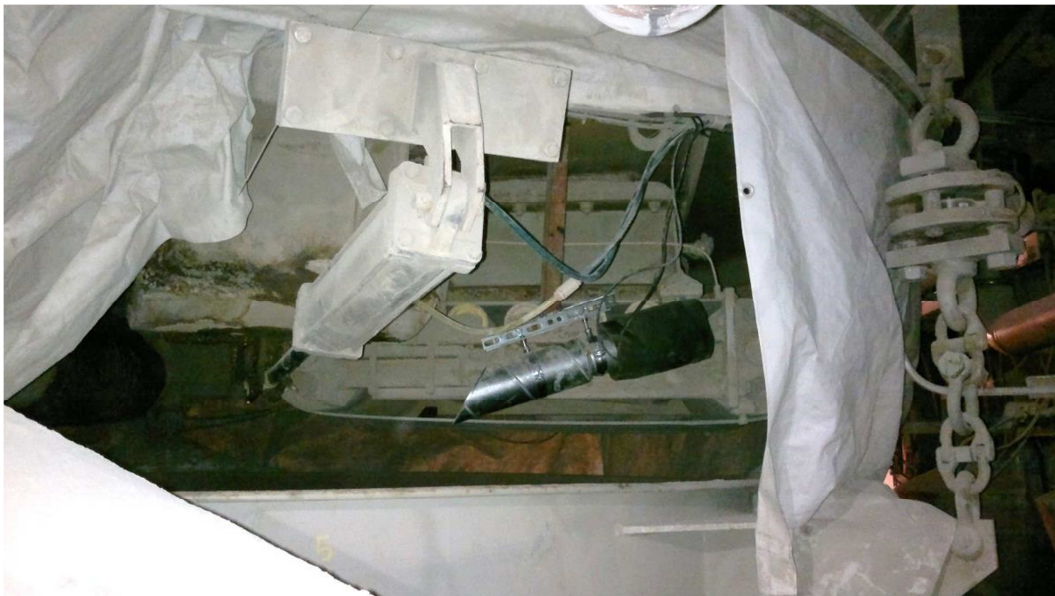
Fig. 2. Moisture sensor installed under a silo hedge door. This sensor is equipped with a heater element.
