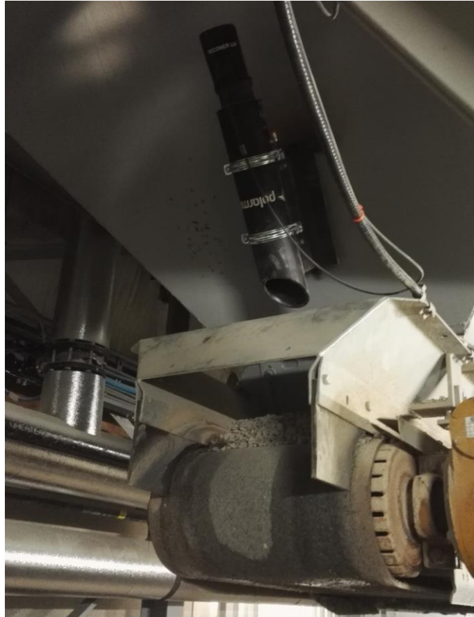
Figure 1. Probe installed over a bin belt feeder.
